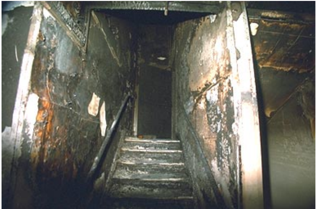
Photo 8. The central stairway was immediately adjacent to the room of origin on the first floor. This stairway was the primary avenue of fire spread to the second floor.
