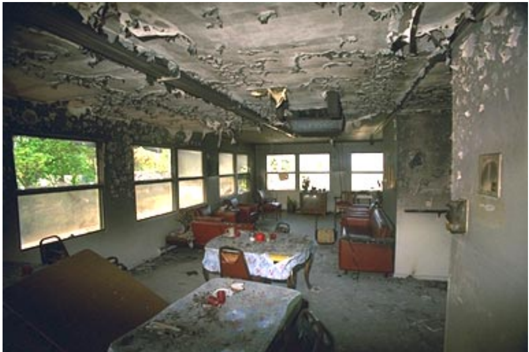
Photo 11. The common room at the south end of the building on the second floor was damaged by the spread of heat and smoke.
