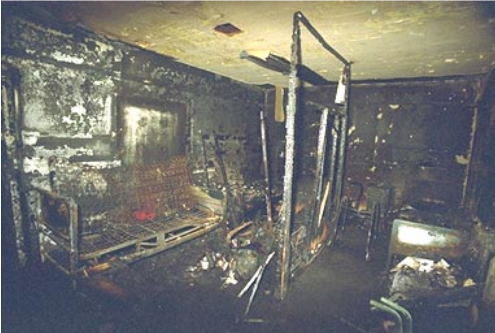
Photo 6. The contents of the room of origin were severely damaged by the fire.
