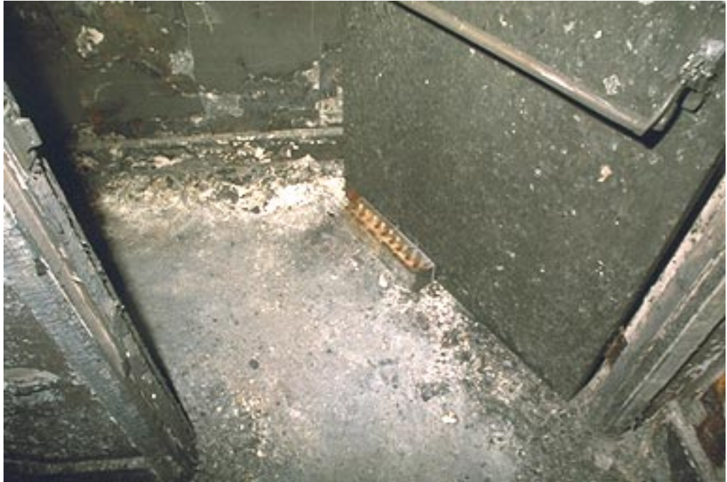
Photo 2. The door on the landing for the central stairway had been propped open at the time of the fire.
