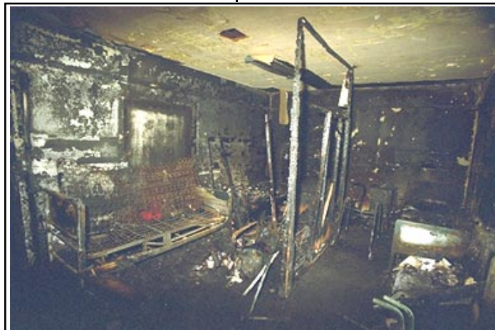
Room of Origin. It was determined that the fire started in the bed.
