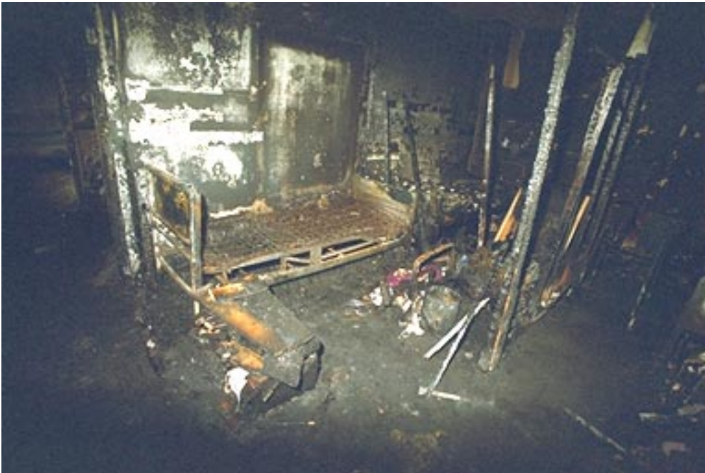
Photo 7. The fire was believed to have started in the area of this bed in Room 1 on the first floor.
