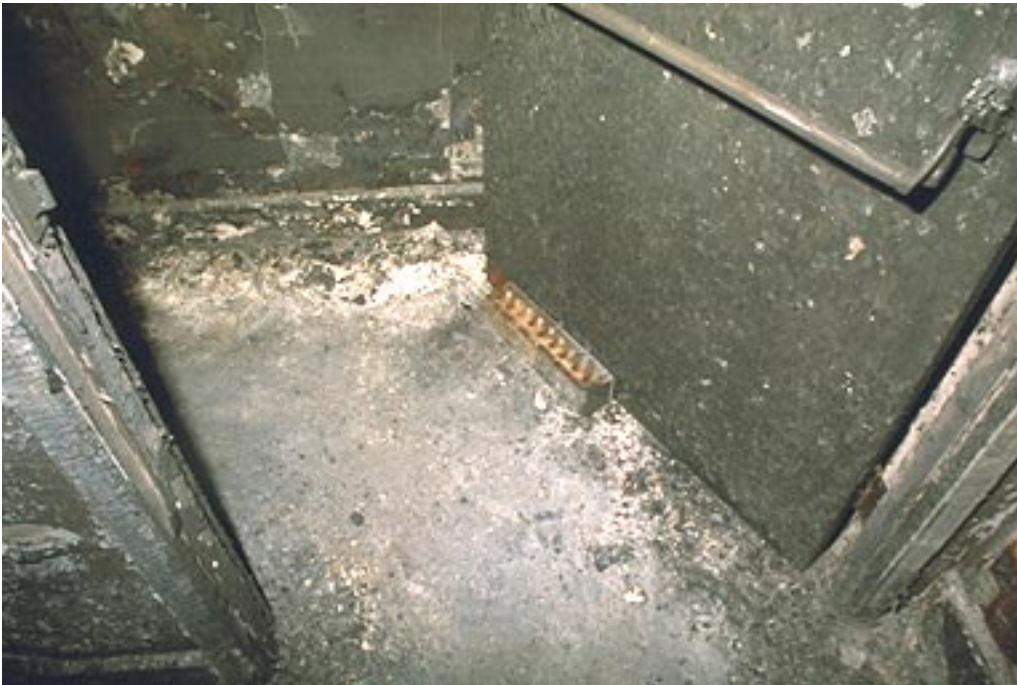
Photo 12. The door leading to the second floor from the central stairway was propped open at the time of the fire.
