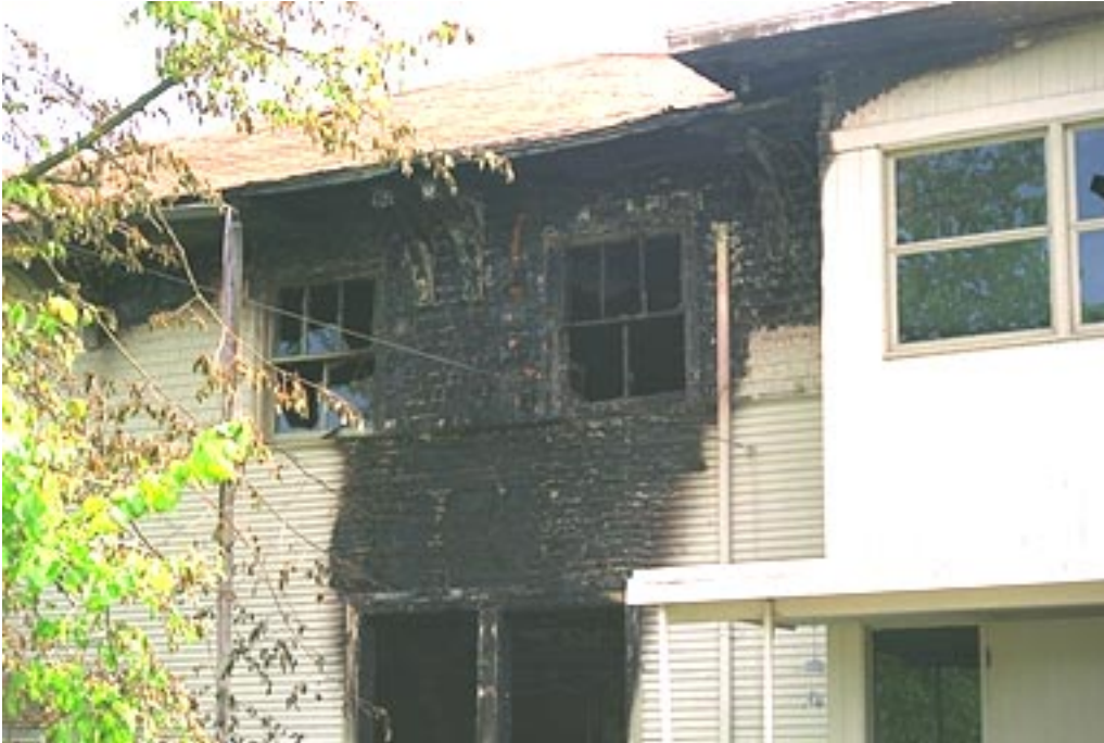
Photo 4. Southwest view of the facility. Although the fire vented out the exterior window on the first floor, there was not any significant fire spread to the second floor from the exterior of the building.
