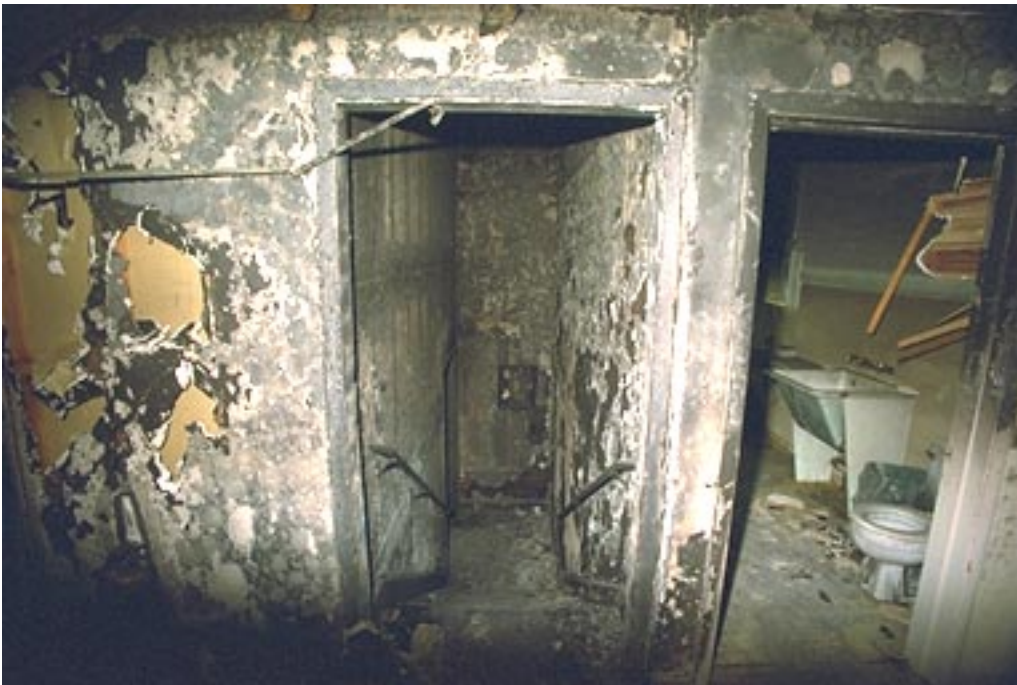
Photo 5. The bathroom where two residents died on the second floor was next to the central stairway that was the main avenue of fire spread to the second floor.
