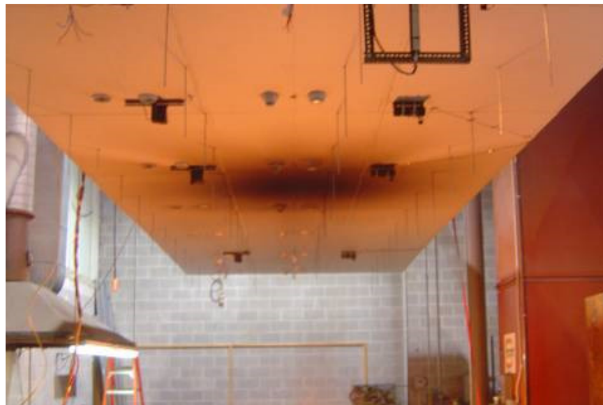
Figure 3-1 – View of HAI movable ceiling
