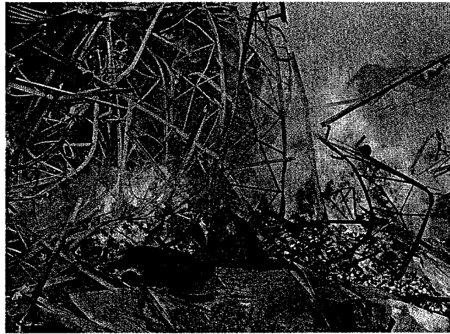
The light metal frames of the fire building's storage racks supported both the stored commodities and the warehouse roof assembly.
